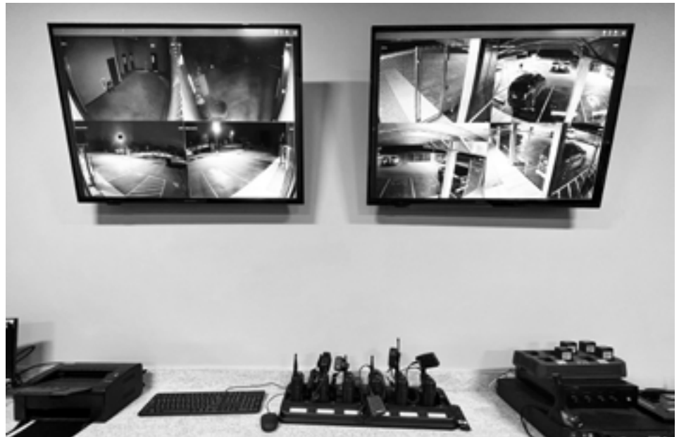
Squadroom monitors allow staff to view activity inside and outside the station.
